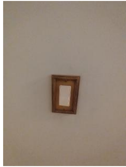
Switch/Outlet Taken on: 2018-10-03 12:30:33 Taken at: 32.76292889, -79.98744807 Image
