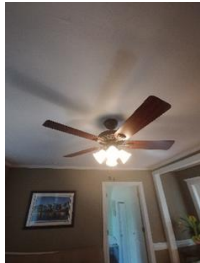
Light Fixture/Fan Taken on: 2018-10-03 12:06:05 Taken at: 32.76305183, -79.98739853 Image
