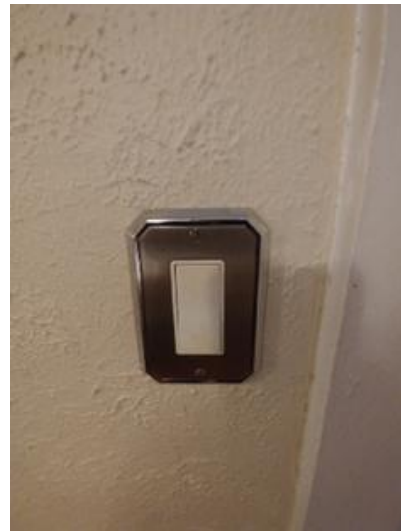
Switch/Outlet Taken on: 2018-10-03 12:22:43 Taken at: 32.7627476817, -79.9872848316 Image
